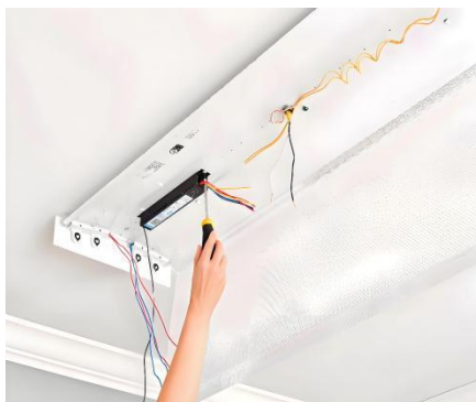
Fluorescent Light Fitting
